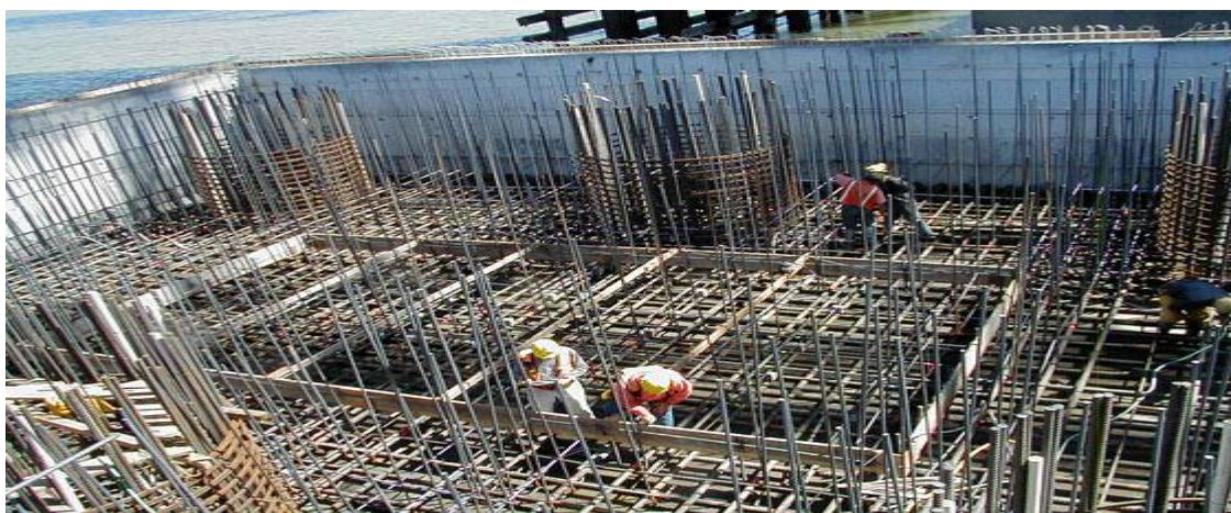
Figure 2-3: Reinforced concrete consists of ordinary concrete reinforced with reinforcement resist tensile stresses
